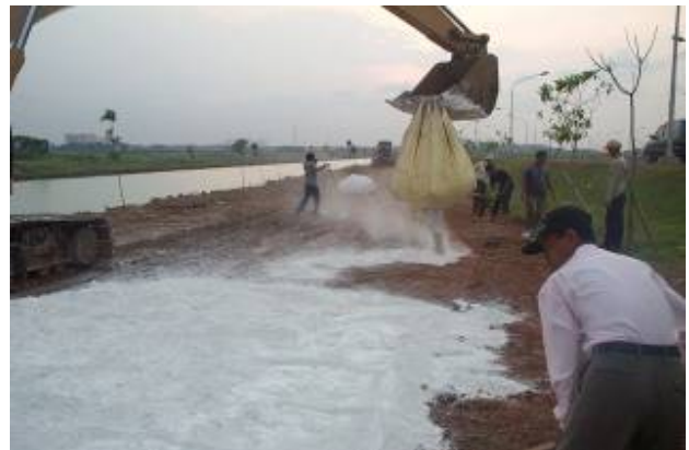
Hydrated Lime spreading
